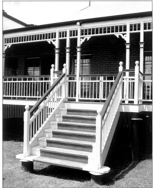
Ant caps provide ground separation for stairs, but regular inspection is required
