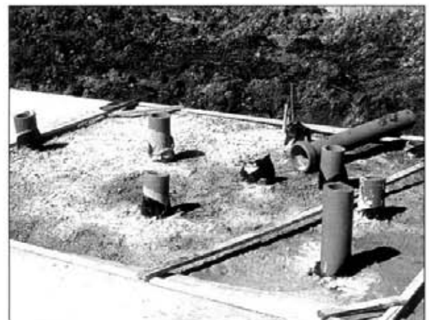
Concrete slab – Special attention to service penetrations and joints is required
