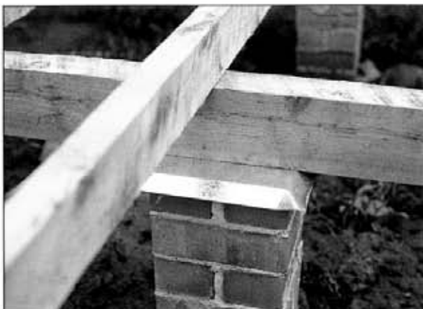
Suspended timber floor detail – Ant capping on brick piers. Regular inspection is necessary
