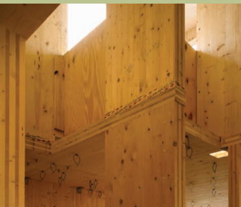
Interior during construction of the Murray Grove Tower Image courtesy of Will Pryce.
